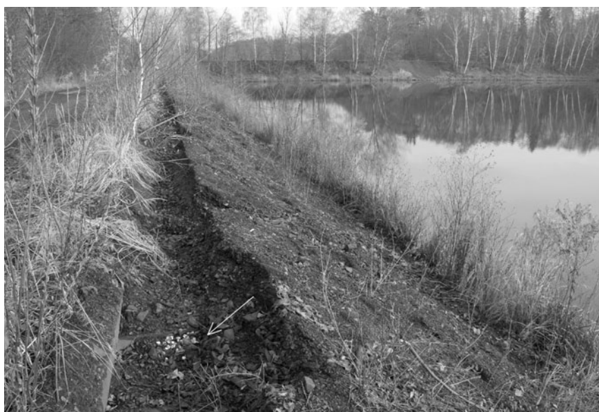
A similar view after the theft of piping from both banks of the reservoir. The white arrow points at a cavity with the dice snake eggshells discovered there (situation as of 6th December 2009)
